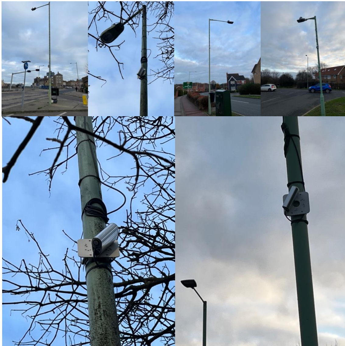
Figure 23: Remote RST Sensors supplied by CIMCON, photographed December 2021 (photo: H Steventon)
