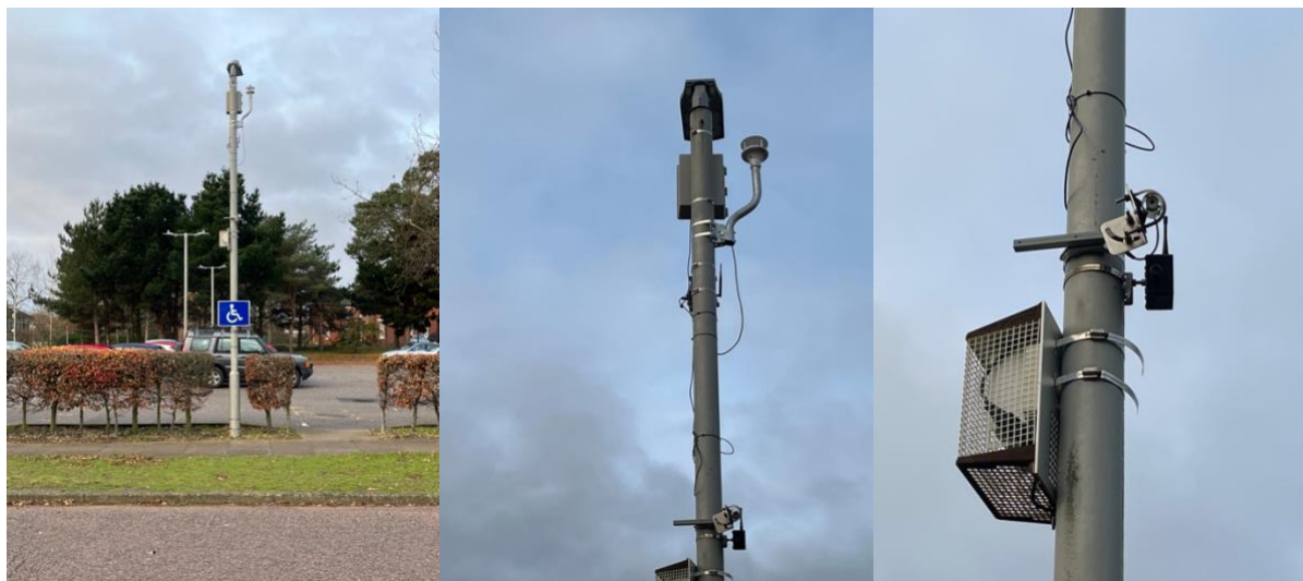
Figure 33: Libelium RST and weather sensor supplied by SSE (photos: H Steventon)
