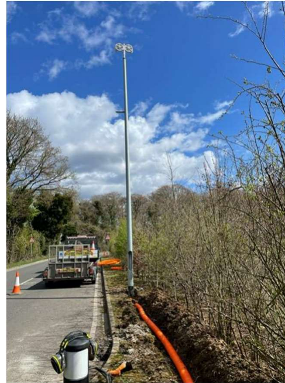
Wind turbine mounted on top of lighting column
