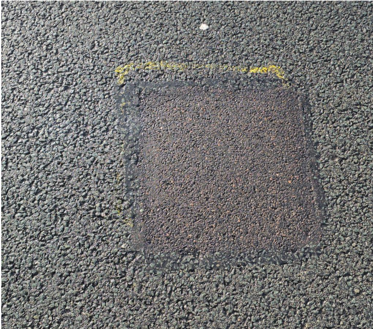
Figure 5 - Phase 2 Pothole Repair Image 3 – EZ Street (Red Stag) – 6 months - Minor deterioration.
