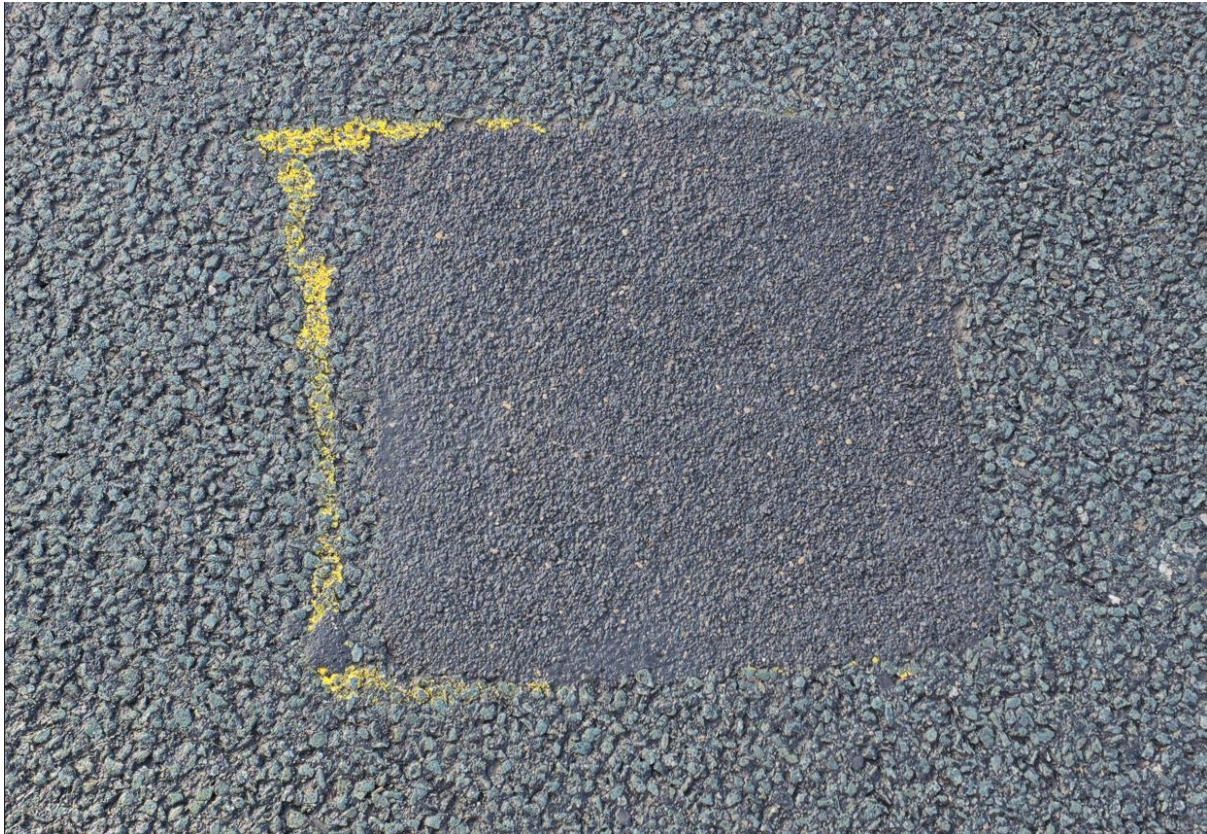
Figure 6 - Phase 2 Pothole Repair Image 4 – Degafill (Degafloor) – 6 months - Minor deterioration.
