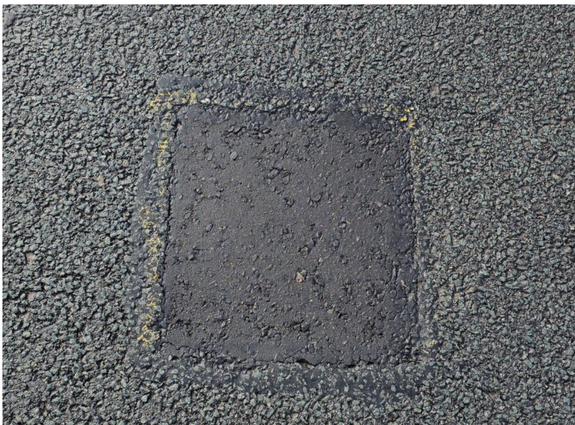
Figure 9 - Phase 2 Pothole Repair Image 7 – HRA 45/10 (MQP) – 6 months – Moderate deterioration.
