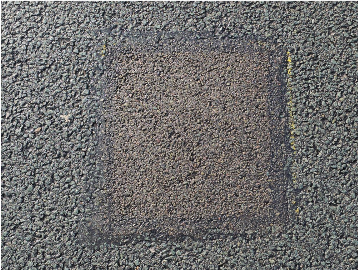
Figure 4 - Phase 2 Pothole Repair Image 2 – Ultipatch Bio (Tarmac) – 6 months - Minor deterioration.
