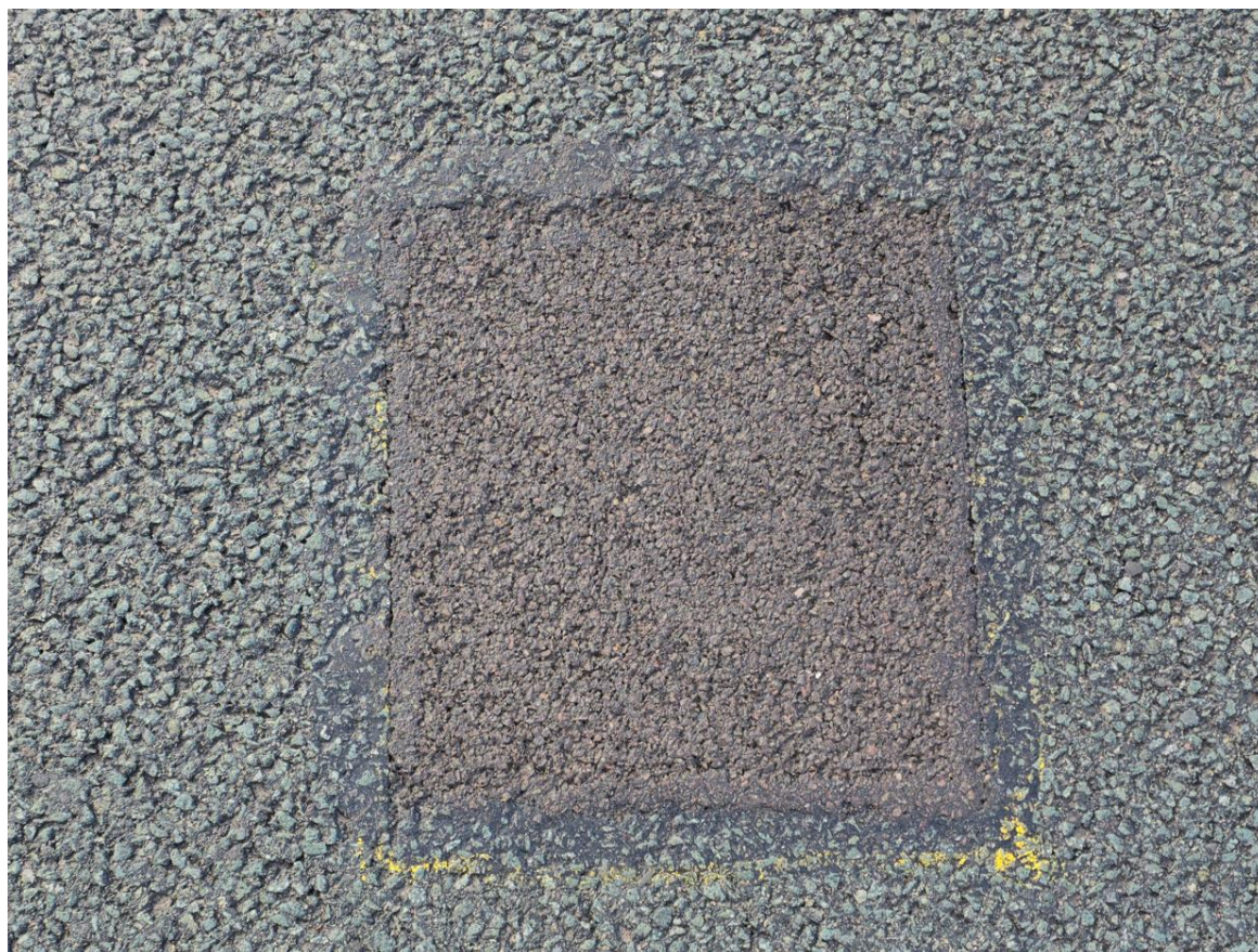
Figure 3 - Phase 2 Pothole Repair Image 1 - Viafix (Viatec) – 6 months - Minor deterioration.
