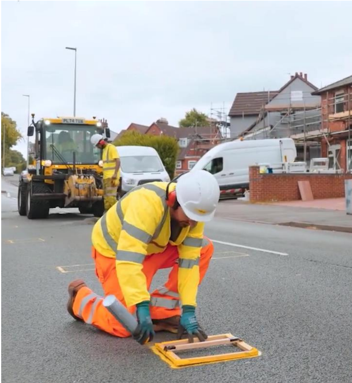
Figure 2 – Image of artificial potholes being marked up on Thimblemill Road.
