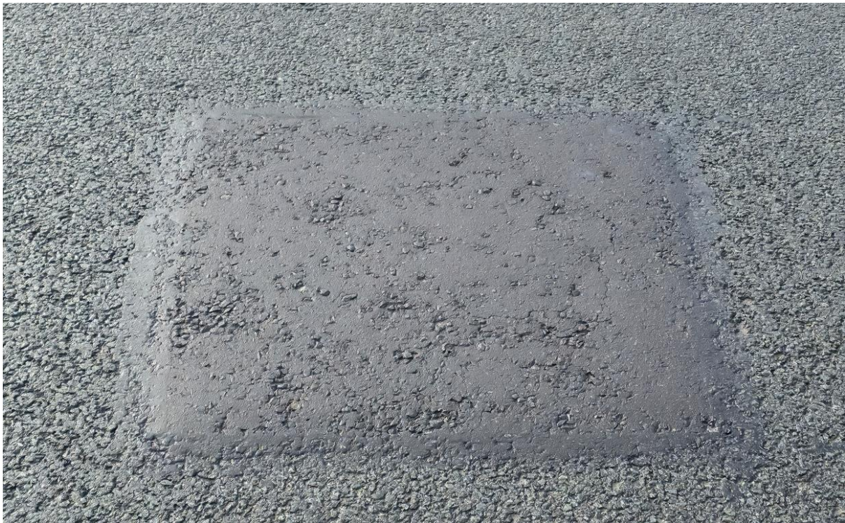
Figure 7 - Phase 2 Pothole Repair Image 5 – Thermal Road Repairs (TRR)– 6 months - Minor deterioration.
