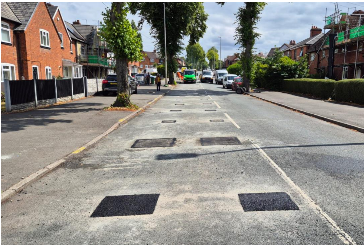
Figure 1 – Image of Thimblemill Lane – Potholes Phase 2.
