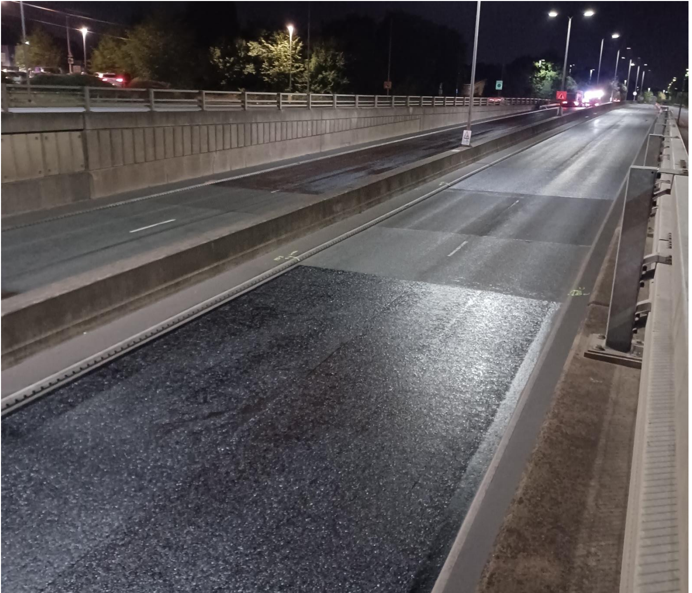
Figure 12 – Image of A41 The Expressway during curing period of Colas Active Sealing.
