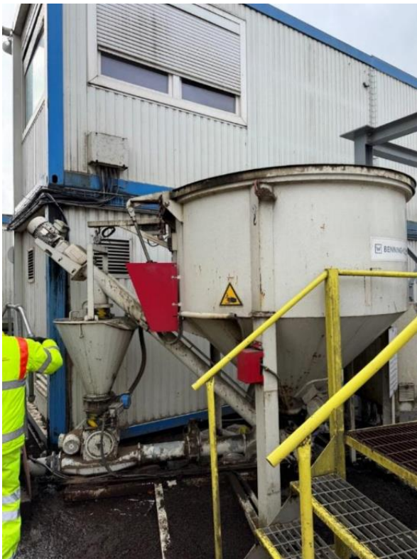
Figure 3: Dosing system with one silo
