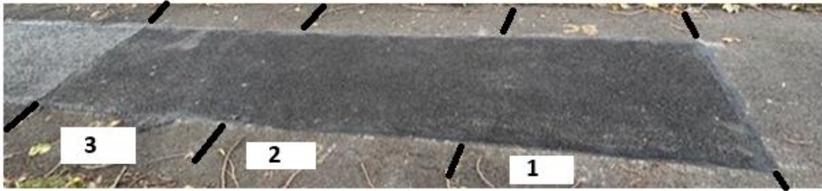
Figure 6. Cycle Path HMA surface conditions
