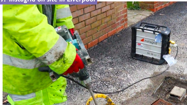
Figure 17: Instagrid on site in Liverpool
